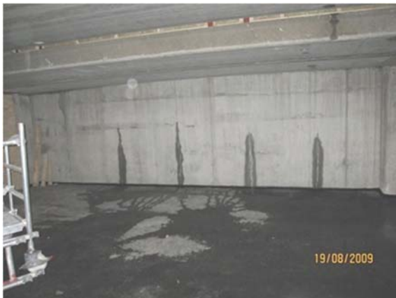
Figure 1 – Example of through-cracking and water leakage in a wall. Photo: B.Kristiansen, AF Gruppen
